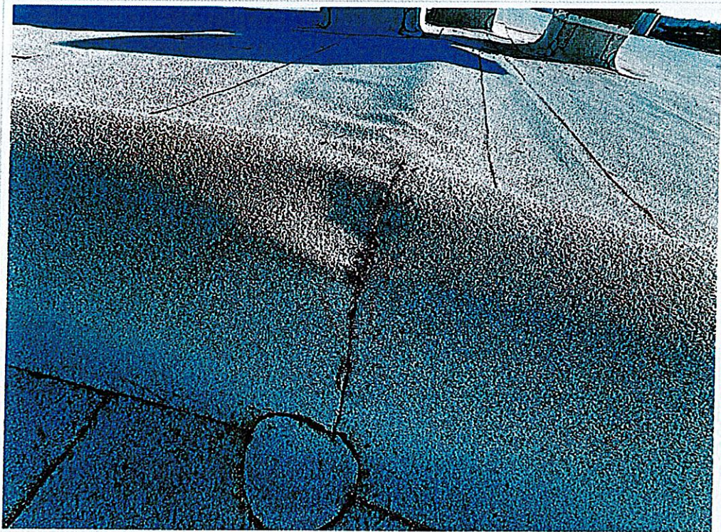
( 1 ) Fish mouth at expansion joint.
